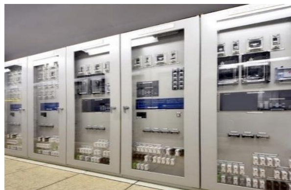
Fig. 1. Typical control cabinets at critical civil infrastructure facilities
